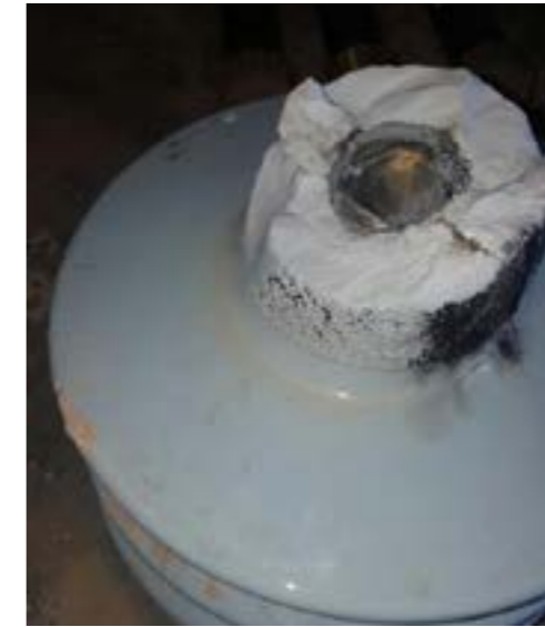
Damaged volt insulator
